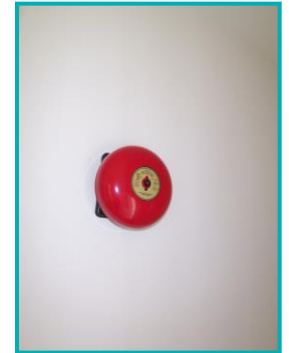
Fire Sprinkler Alarm
