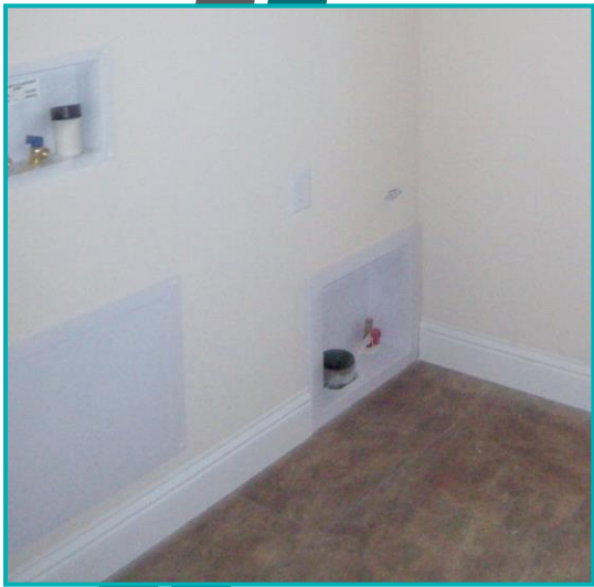
Plumb for Gas Dryer
