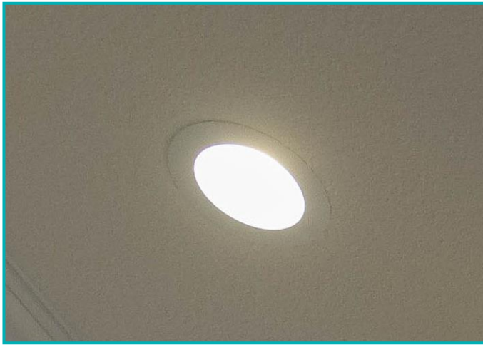
(STD) 4" LED Can Light (1) each room and above kitchen sink
