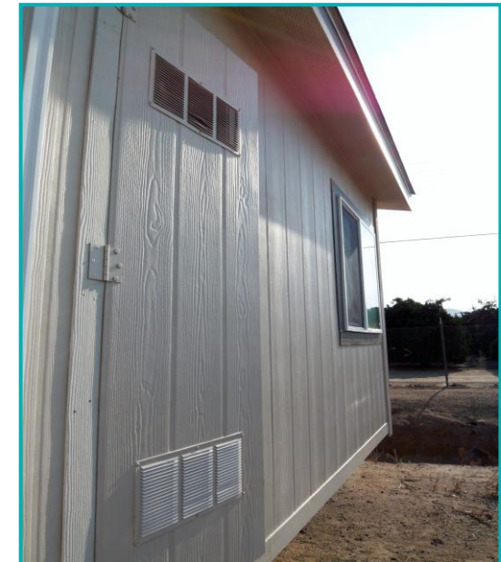
Cement Water Heater Door
