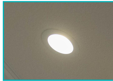
Bathroom Ceiling light
