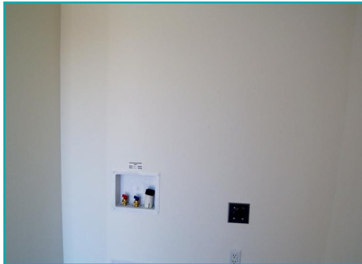
Plumbing for Washer and Electric Dryer
