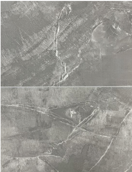
15"x26" Cracked Slate
